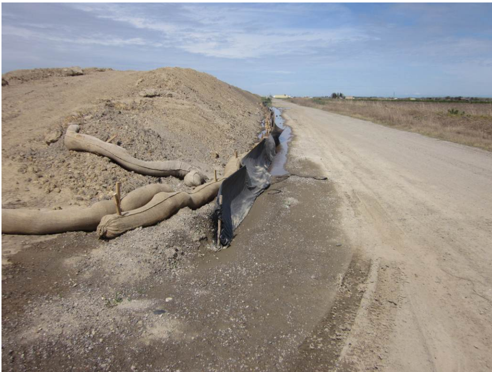
Photo 4: Silt fence and fiber roll placed along the edge of the soil stockpile adjacent to McAusland Road. These BMPs were recently repaired/replaced based on site observations by the project QSP/QSD.
