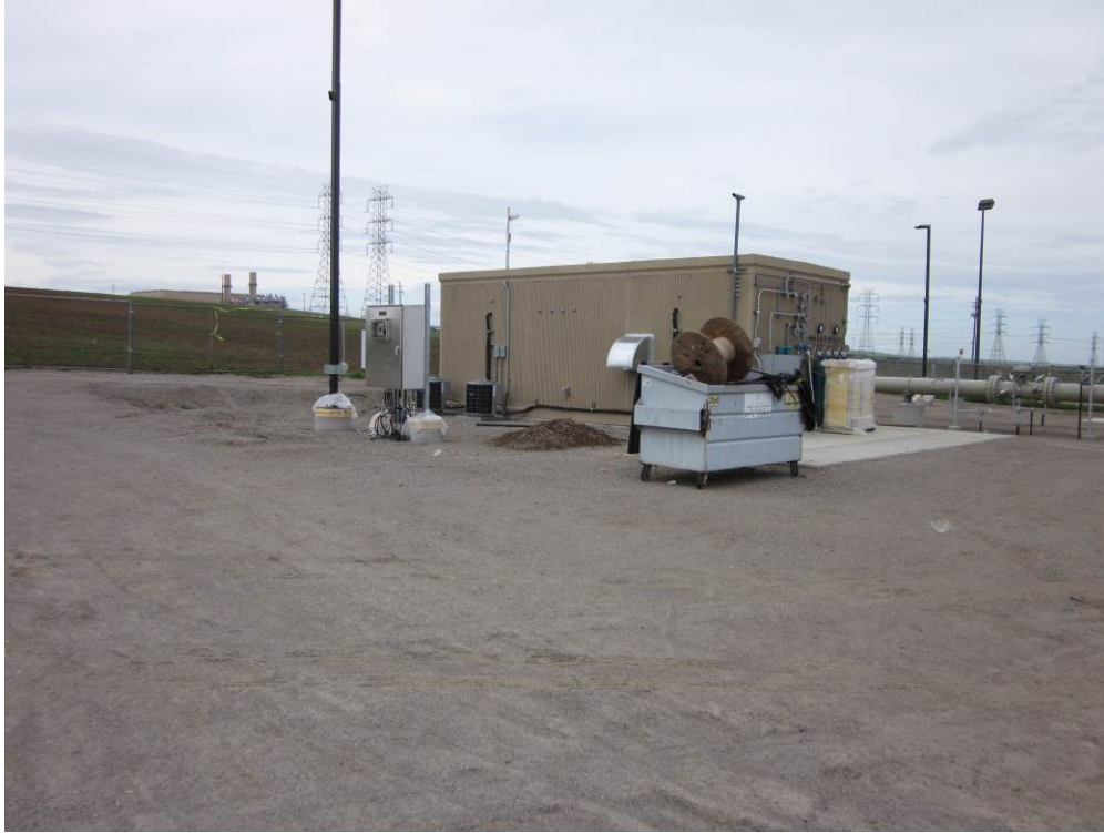
Photo 5: Electrical tie-in work underway at the Metering Station site. Final grading of the site is almost complete and construction debris has been mostly removed.
