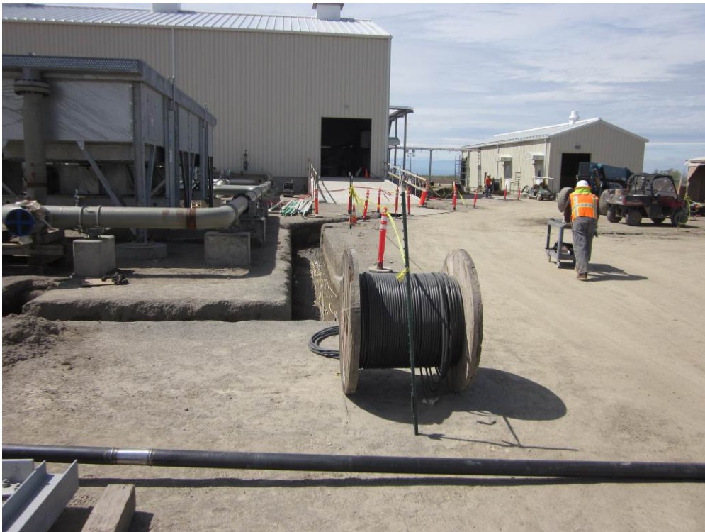
Photo 2: Open electrical line trenches to facilitate electrical work near the compressor building and utility building at the Compressor Station site.
