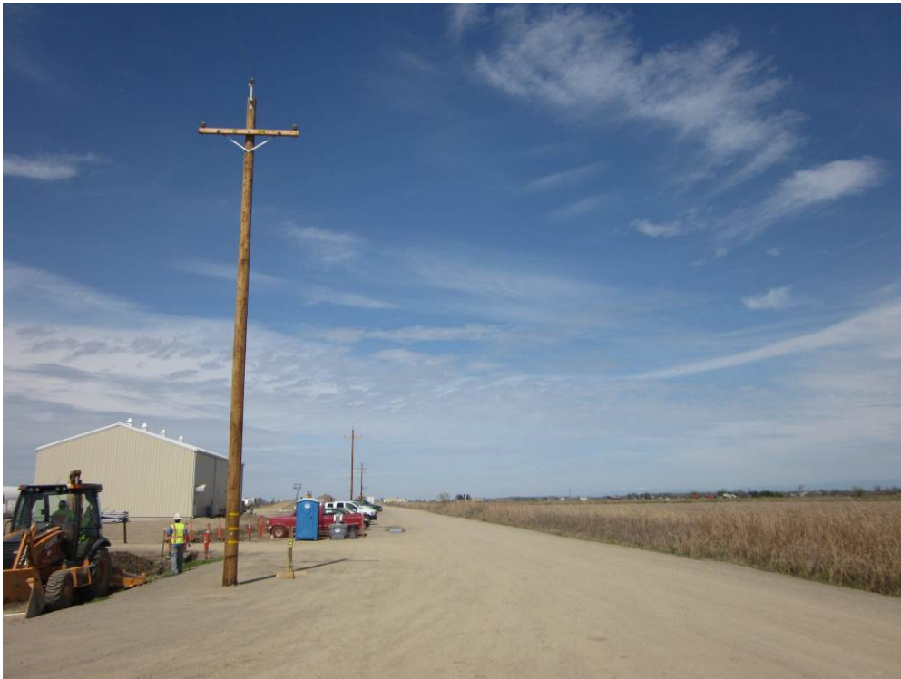
Photo 6: PG&E electrical lines along McAusland Road to be used for toe-in to the electric utility meter at the north end of the Compressor Station site.
